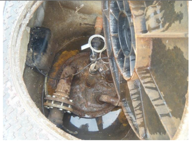
Cuve enterrée GNR (10m 3 )
